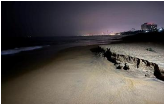
Figure I: Severe erosion close to the Barracuda restaurant
